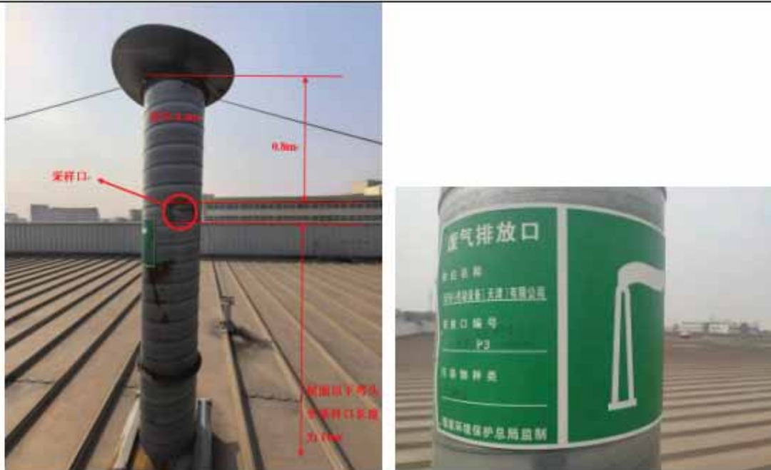
废液间废气排气筒 DA005
