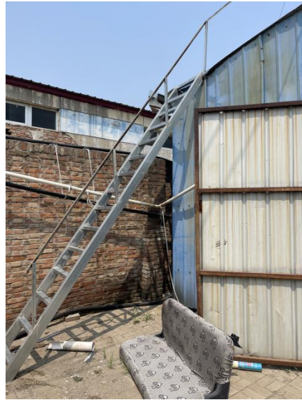
废气排放检测口便梯
